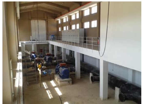
PUMPING STATION 2500m 3 / h WITH POSSIBILITY OF EXTENSION TO 5000m 3 / h
