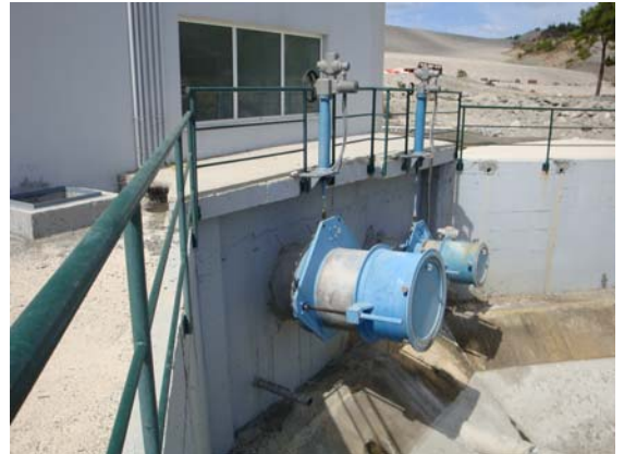
BARRIER EVACUATOR AND ECOLOGICAL SUPPLY
