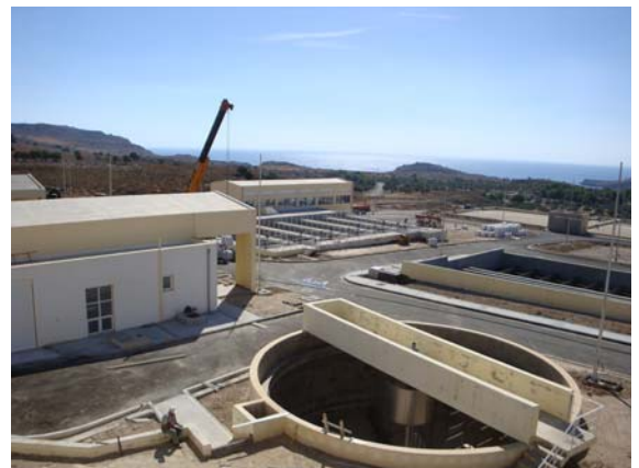
WATER TREATMENT PLANT - RHODES
